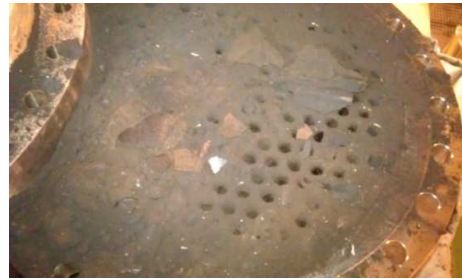
Top of #1 Heater in the Torrefaction Loop. Significant deposits caused blockage and required cleaning after 4 to 7 days of operation.
