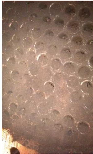
Photo of the inlet tube sheet on the condenser during later part of 2012
